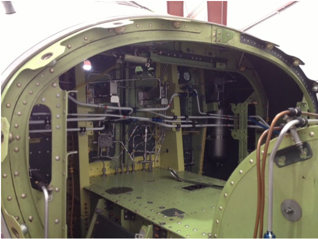
This is where the SyberVision™ LRUs will be installed to support the next generation cockpit for the SJ30.
